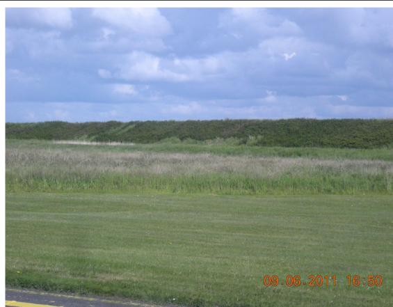
Photo 6: Major Shannon tidal embankment adjacent to the airport road towards the eastern end of the airport.
