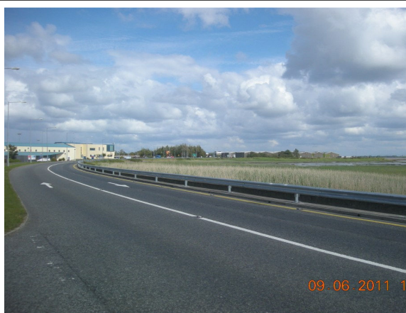
Photo 5: Access road along the top of the embankment bordering the Shannon Estuary inter-tidal-zone. The Shannon Estuary inter-tidal zone is seen beyond the crash barrier.
