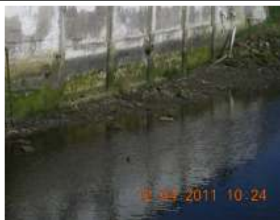
Photo 2: Immediately North on the RHS d/s of Ballylongford Bridge a number of un-flapped valves/outfalls
